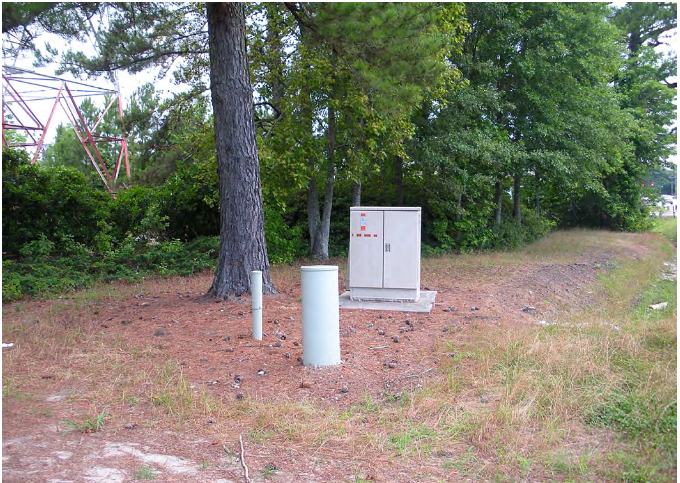
Telephone facilities (outside of compound)
