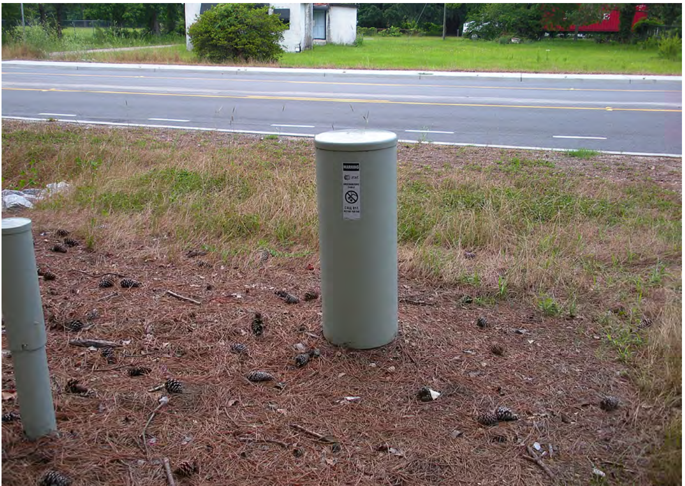
Telephone facilities (AT&T)
